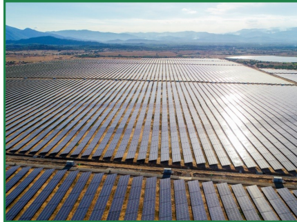
330MW Solar Farm Ninh Thuan, Vietnam
