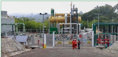
3.6 MW Mindanao 3 Binary Project Kidapawan City, Cotabato
