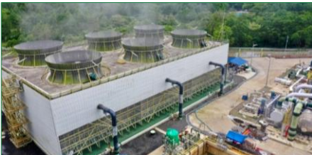
28.9 MW Palayan Bayan Binary Project (Steamfield), Albay
