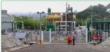
3.6 MW Mindanao 3 Binary Project Kidapawan City, Cotabato
