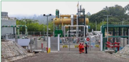
3.6 MW Mindanao 3 Binary Project Kidapawan City, Cotabato
